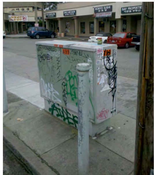
A utility box welcomes neighborhood blight
